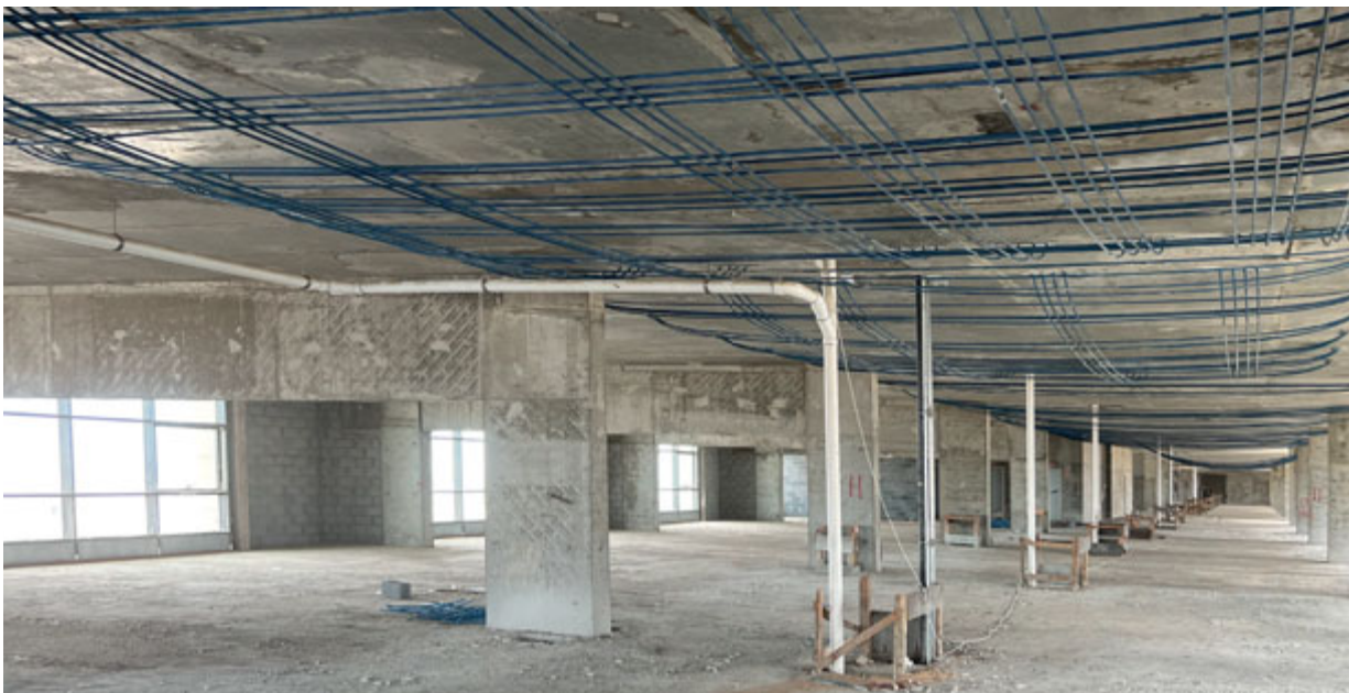
The Khurais Hospital in Riyadh is a former hotel being repurposed. The structure, including floors, needs strengthening using multiple BBR PT MRR solutions to accommodate this change of use. External PT strengthens floor slabs to take the weight of hospital beds and equipment. You can read the full story on page 82.
