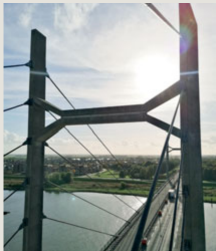
The bridge will require further investigation, as the initial inspection showed corrosion in two locations at the forks' anchor points.
