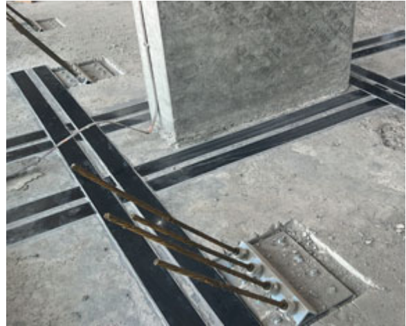
CFRP strips were secured next to columns to help reduce the risk of punching through. The anchorage and tail of the PT tendons used to prevent floor slab deflection can also be seen.
