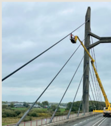
The bridge was built in 1983 and was last inspected in 2014. During October 2022, the De Vries VSL team inspected the 48 BBR HiAm CONA stay cables, which showed that the bridge has deteriorated, and the team advised on how to preserve the corroded steel.
