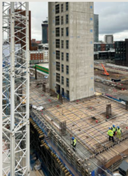
This mixed-use development at First Street in the city of Manchester involved the design and construction of bonded PT floor slabs for three, slip-formed core towers of between 22 and 45 stories. This reduced cycle times, floor-to-floor, and brought down slab thickness and passive reinforcement. We achieved significant programme savings in the frame construction and ensured minimal environmental impact.
