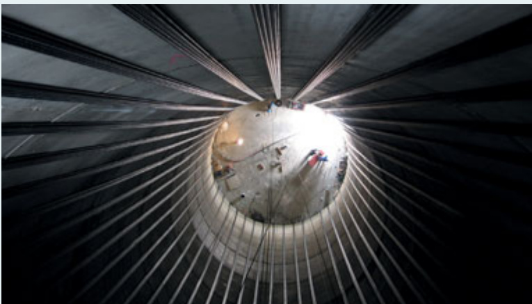
The concrete tower element is stiffened using external PT, reducing the materials required, specifically concrete and cement, high carbon emitters.
