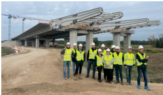
Network Members tour BBR Polska's post-tensioning work on the Warszawa Kukuryki bridge.
