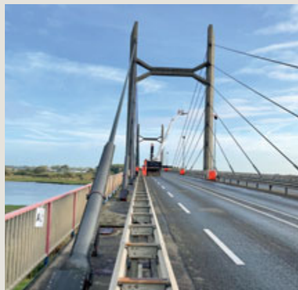
The Molenbrug Bridge over the River IJssel is a vital link between the towns of Kampen and IJsselmuiden, 100km east of Amsterdam, in the Netherlands. The Rijkswaterstaat (Ministry of Infrastructure and Water Management) commissioned De Vries VSP to inspect the BBR system cable-stays.
