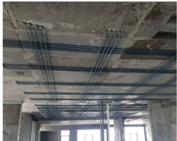
PT tendons on the underside of slab before finishing. These are designed to prevent deflection of the floor/ceiling slab when under load from the floor above.
