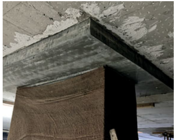
The drop panels of the columns were re-capped and the columns reinforced with rebar then jacketed with a thicker concrete layer.
