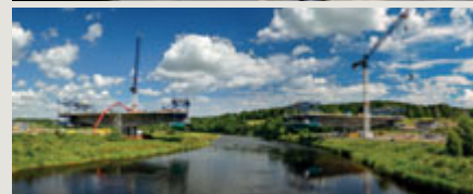
For this balanced cantilever bridge carrying the A90 from Milltimber to Cookney in Scotland, the contractors chose a post-tensioned box girder. This minimized disruption (formwork or piling) to the protected salmon stream in the River Dee flowing below.
